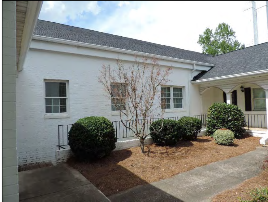
Figure 78: New Hope Presbyterian Church, facing northeast to south side elevation of Education Building
